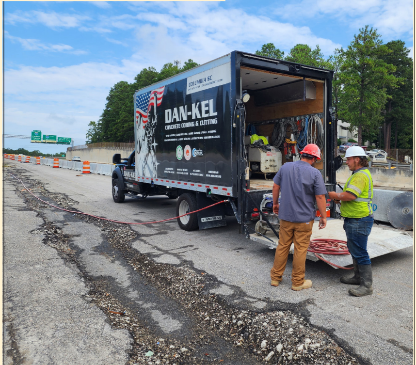
DAN-KEL Concrete Coring & Cutting, saw-cutting pavement along I-126 Median near Colonial Life Blvd.
